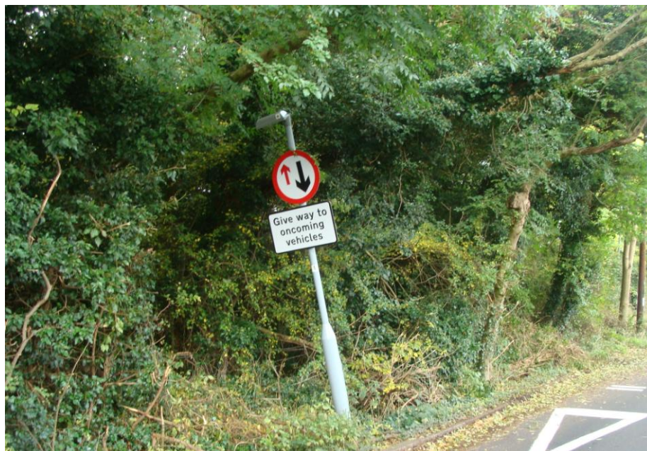
Picture 29. Re-erection of this street sign would a make worthwhile albeit minor visual improvement. Issue now resolved
